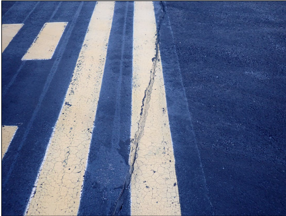
TW-01-08: L&T Cracking
