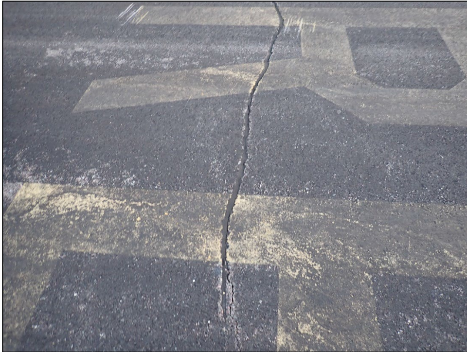
AP-01-08: L&T Cracking
