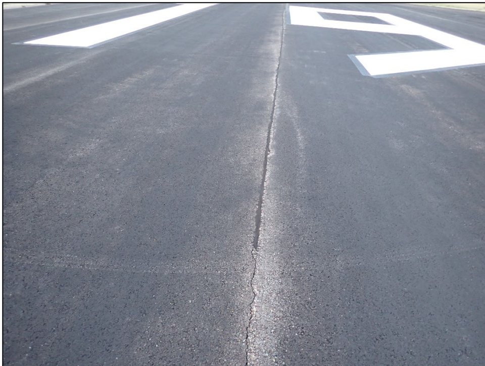
RW01-01-62: L&T Cracking
